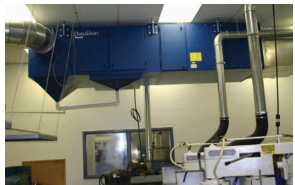
Modular Mediafilter™ on Grinding 2,000 cfm (3,397 m 3 /h)
