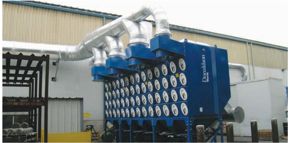
DFO on Grinding 74,000 cfm (125,700 m 3 /h)
