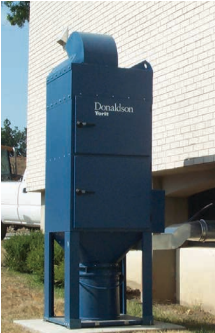
UMA - School Wood Shop 2,000 cfm (3,397 m 3 /h)
