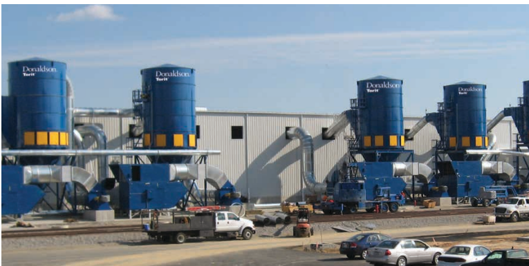
RF - Wood Furniture Facility 403,000 cfm (684,556 m 3 /h)
