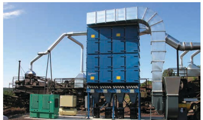
DLMC on Rock Crushing 41,000 cfm (69,645 m 3 /h)
